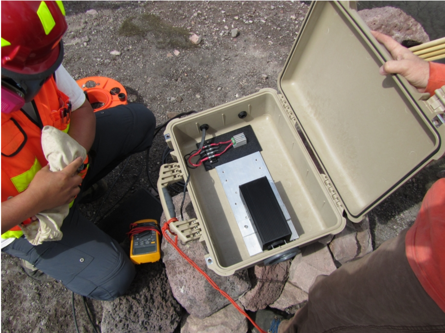
Camera in Pelican case, attached to aluminum baseplate
